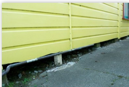
Figure 7: Areas of subfloor space with insufficient clearance
