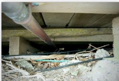
Figure 8: Areas of subfloor space with insufficient clearance
